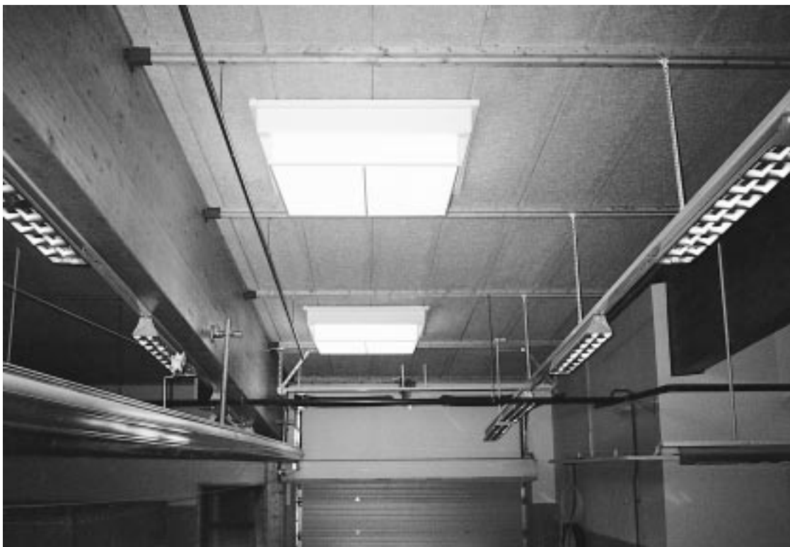
Figure 2: Ceiling view of the daylight system showing the opalescent light fittings
